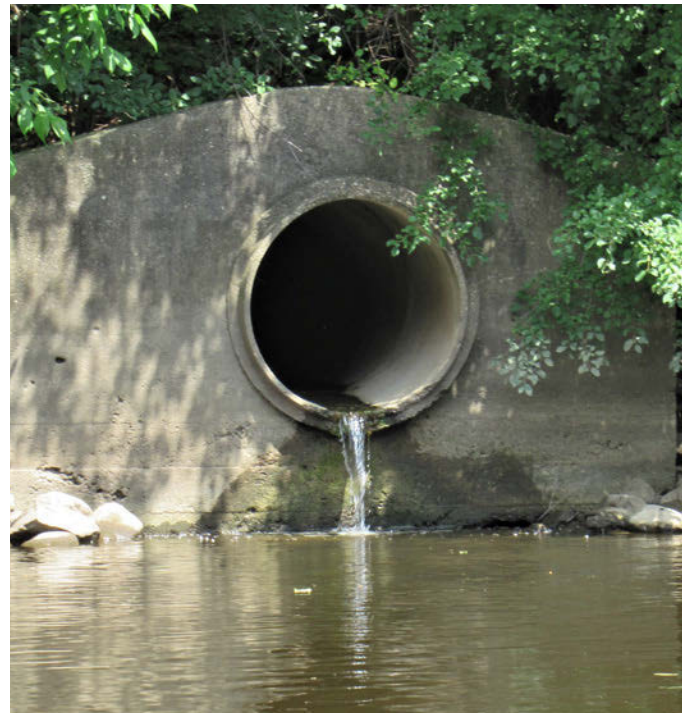
Pipe part of a combined sewer overflow system in Lansing.
