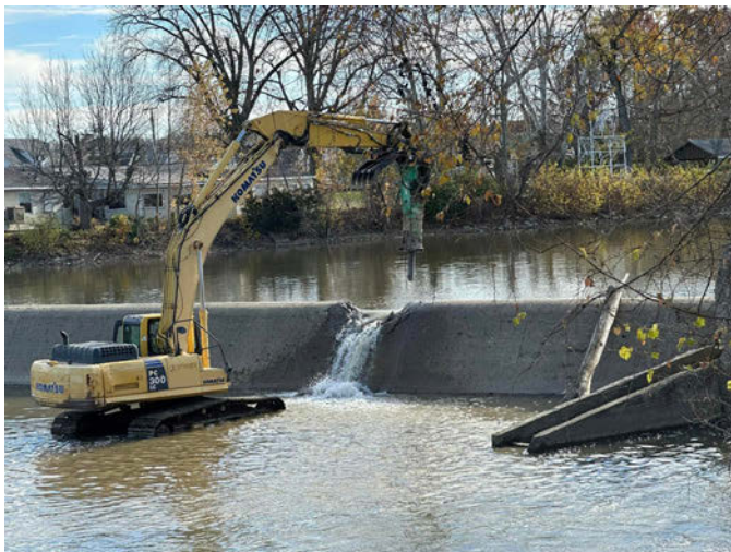
Heavy equipment breaking down the Charles Mill Dam. Credit: EcoSystems Connections Institute, LLC
